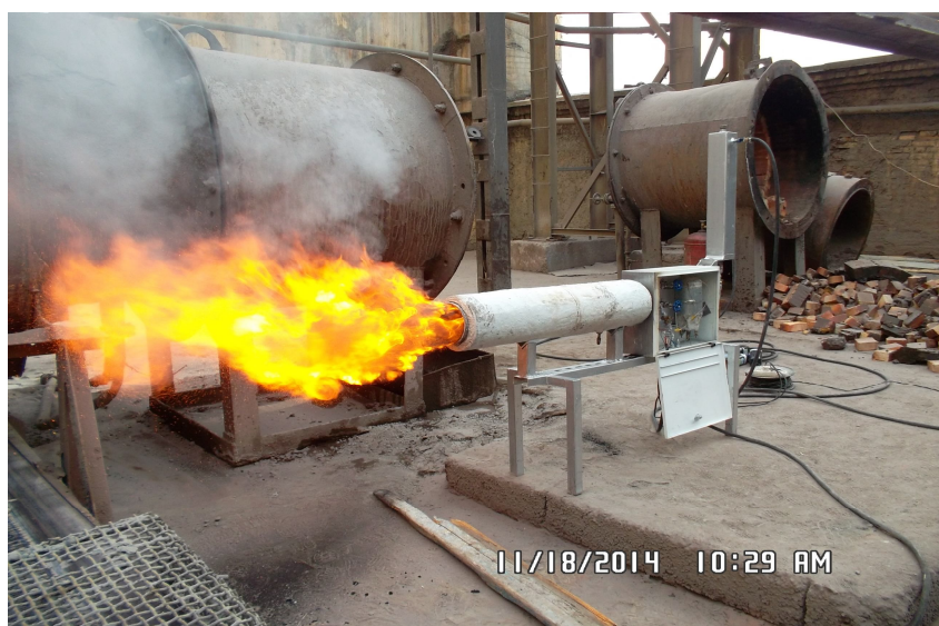
Fig.9. Combustion of WCFS in furnace aggregate of oven dryer of Angren SC “Almalyk MMC” with using of jumbo burner with power 100 Kw/h
