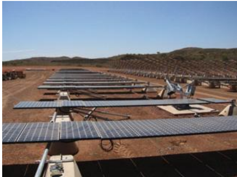
Fig.1.2.8. Combined diesel-solar power plant
