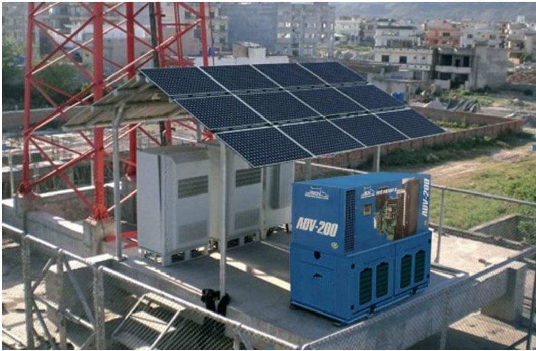
Fig.1.2.11. Solar battery + inverter + DGS+ management system
