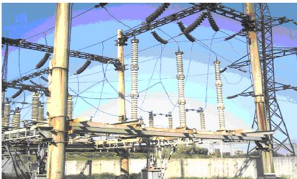
68-rasm. Izolyatorlar shodasining ko'rinishi
