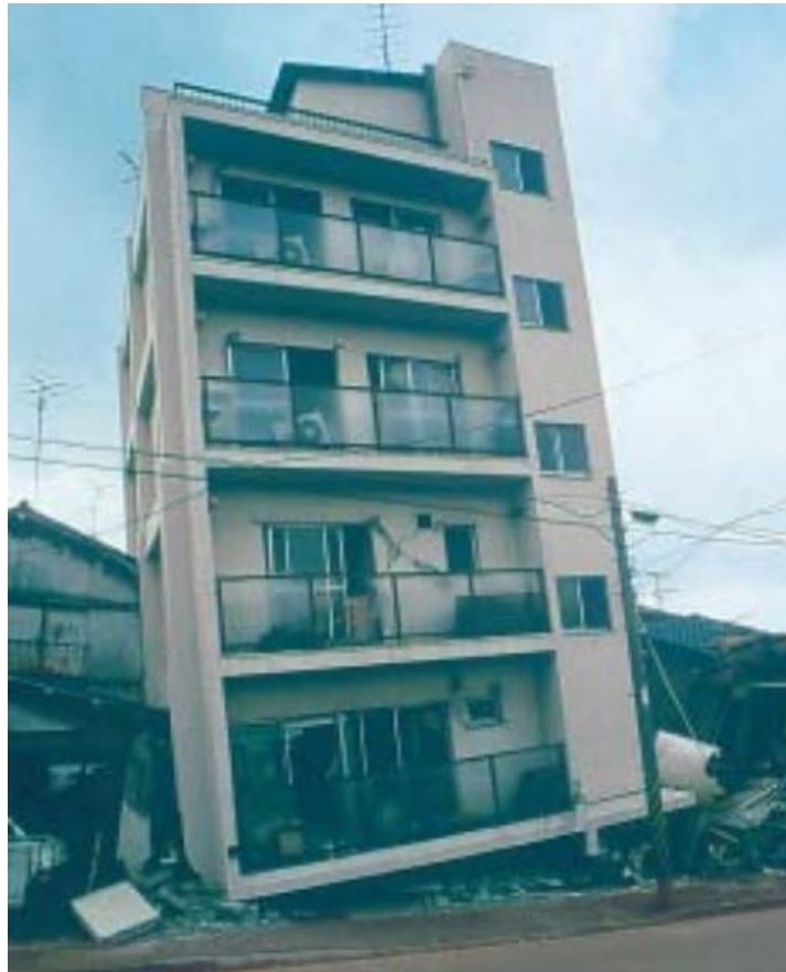
Figure 9.4. The well-braced upper part of the building collapsed onto the ground floor
