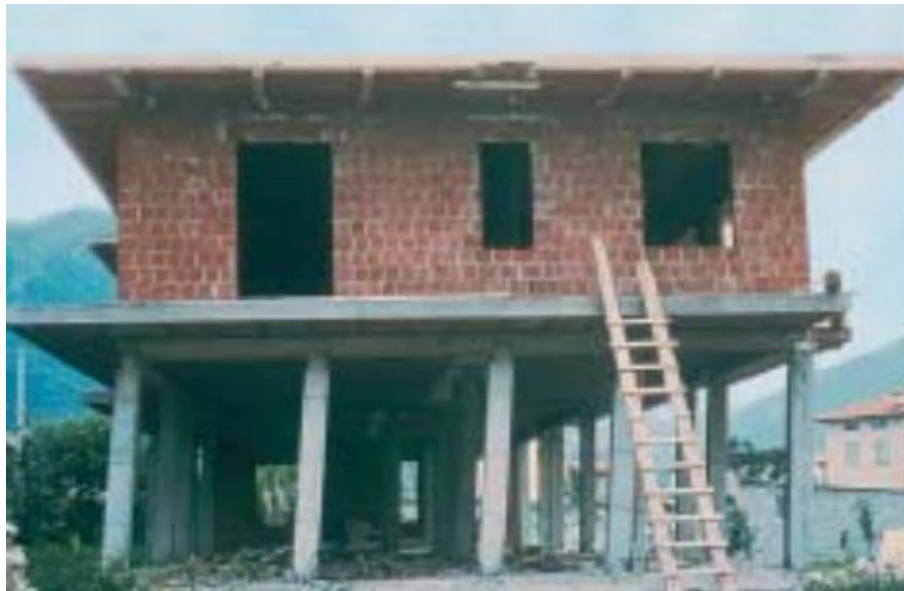
Figure 9.1. This sway mechanism in the ground floor of a building under construction almost provoked a collapse (Friaul, Italy 1976).
