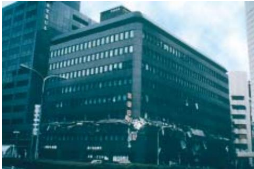
Figure 9.8. In this commercial building the third floor has disappeared and the floors above have collapsed onto it (Kobe, Japan 1995).
