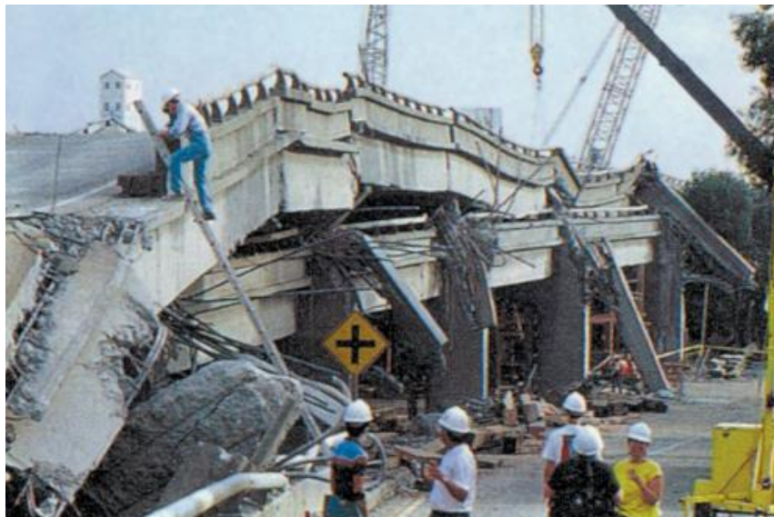
Figure 3.1 A part of the Cypress Freeway in Oakland California that collapsed during the 1989 Loma Prieta earthquake.
