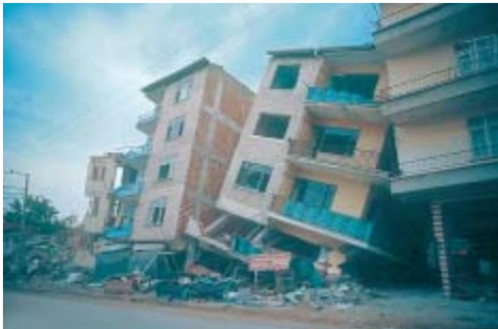
Figure 9.2. Sway mechanisms are often inevitable with soft storey ground floors (Izmit, Turkey 1999).
