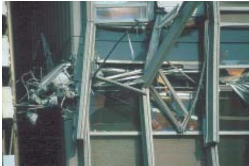
Figure 9.10. This close-up view shows the crushed upper floor of the office building (Kobe, Japan 1995).
