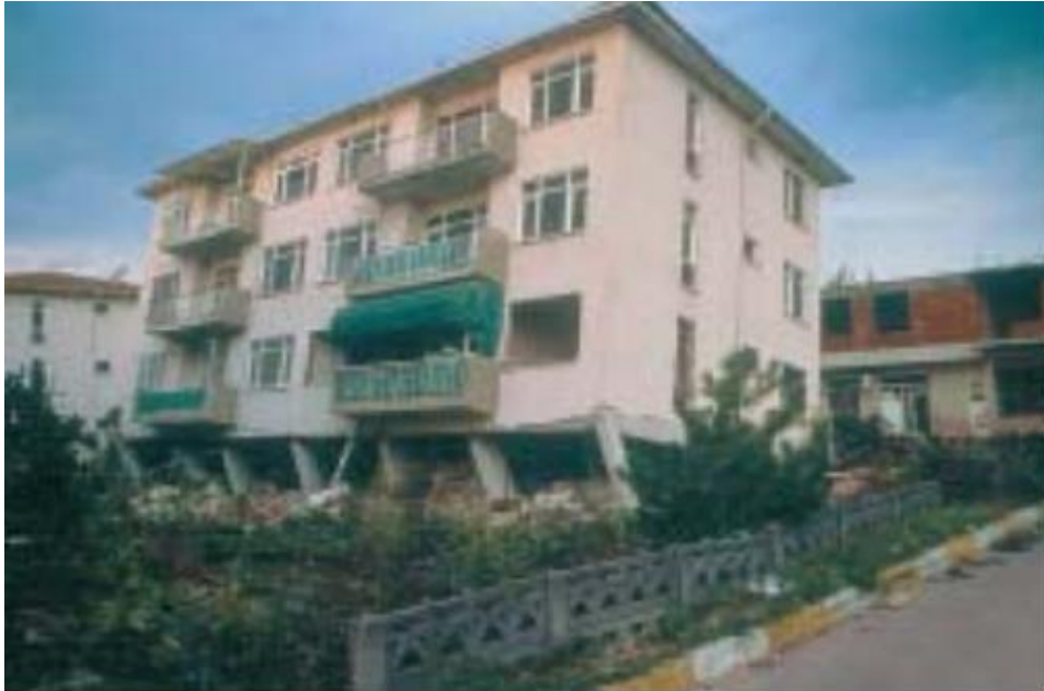
Figure 9.3. Here the front columns are inclined in their weaker direction, the rear columns have failed completely (Izmit, Turkey 1999).
