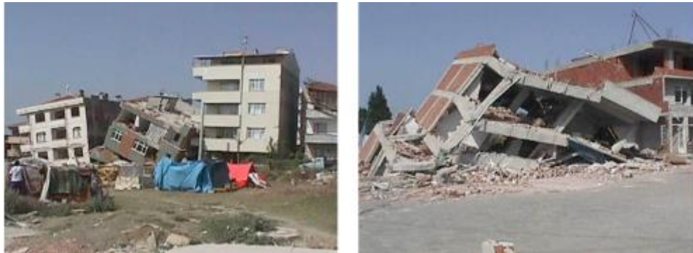
Figure 3.2 Buildings damaged by the 1999 earthquake in the Izmit area, Turkey.
