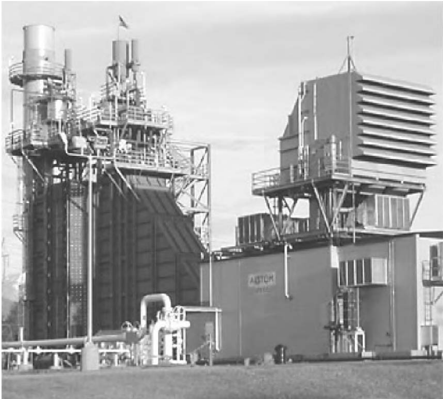
Figure 2-20. Combustion turbine power plant.
