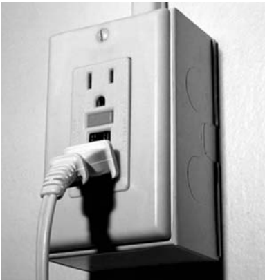
Figure 10-13. Safety hazards at home. Always be vigilant about electrical safety at home!
