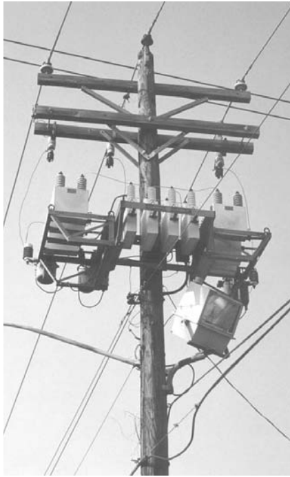
Figure 4-40. Distribution capacitor bank.
