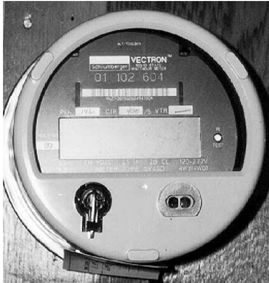
Figure 6-7. Solid-state kWh meter.
