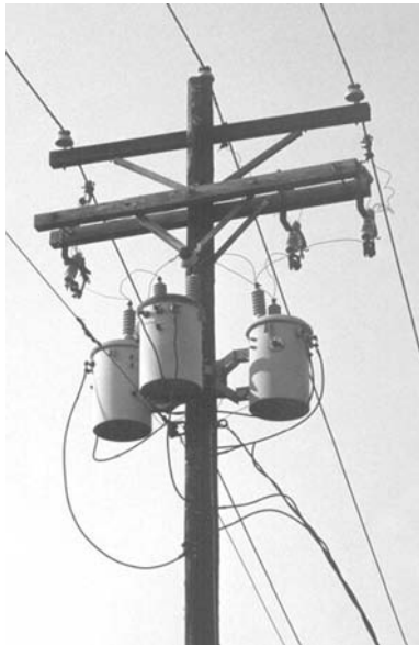
Figure 5-18. Three-phase transformer bank.
