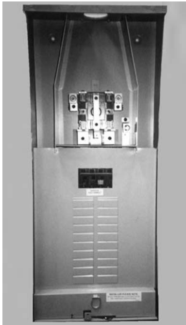
Figure 6-13. Meter cover removed.
