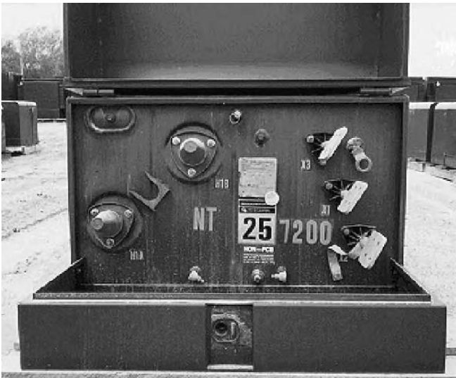
Figure 5-34. Switching transformer. Courtesy of Alliant Energy.
