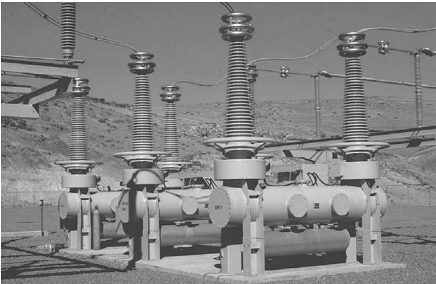
Figure 4-26. 345 kV Gas breaker.
